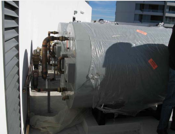
Hot water storage of cogen unit
