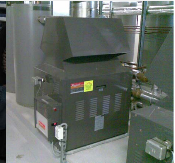
Raypak gas boilers
